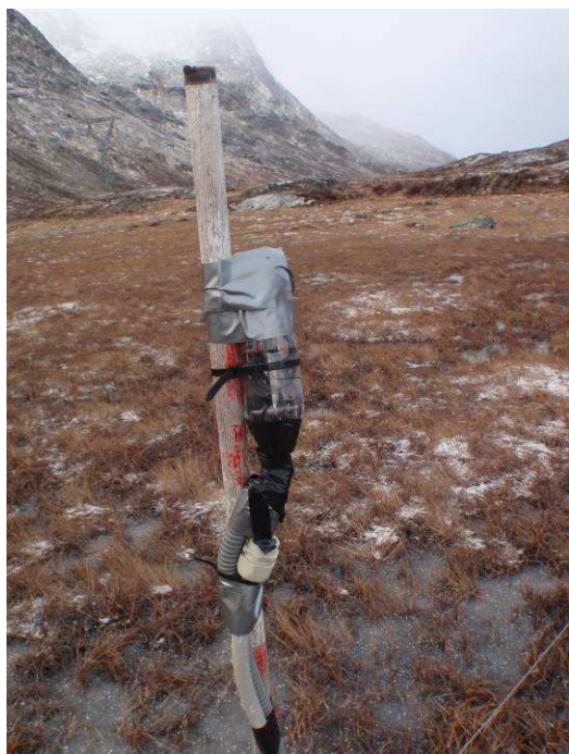
Power cables still “hot” powering Interact Fen
