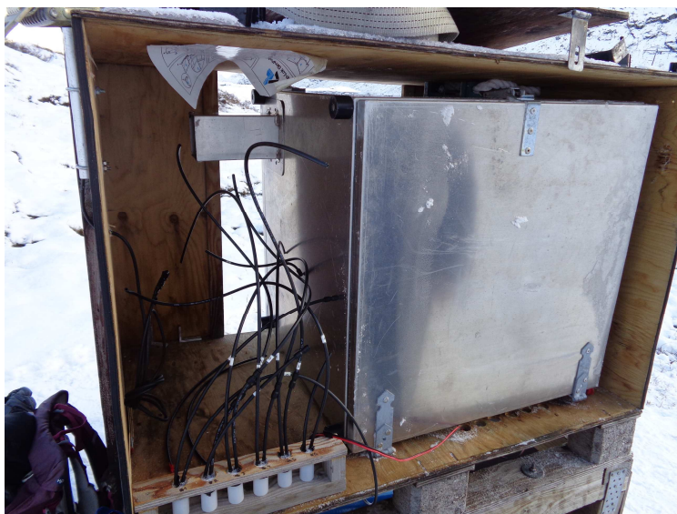
Enclosure inside the Methane hut
