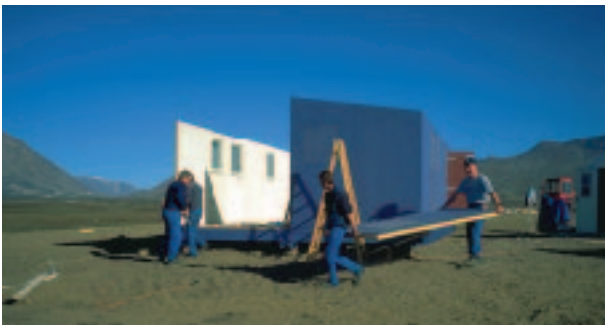
The four construction workers from 'Venslev Cabins' at the chores of erecting the five buildings.
