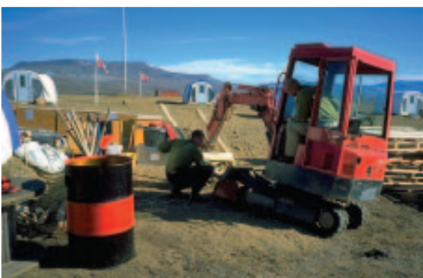
The 'mini' excavator proved indispensable in many situations from digging to fork-lifting.
