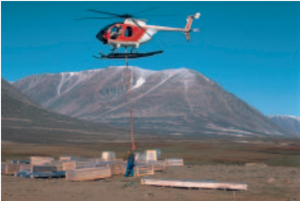
Starting 10 August the Hughes 500 helicopter unloaded 120 slings of building materials at the construction sites.
