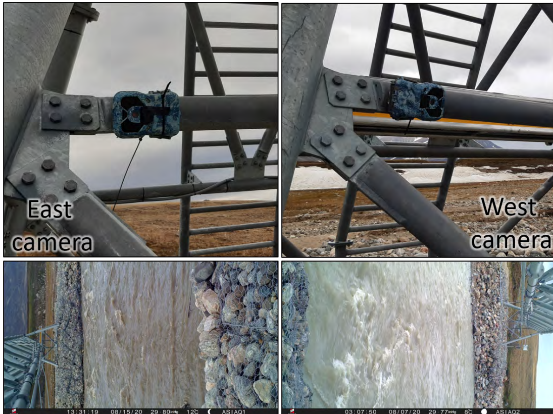
Figure 51: Camera mountings and frames for the time lapse cameras on the bridge.
